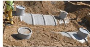
3-Underground Water Tank
